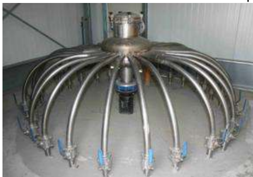
Hydraulic mixing system
