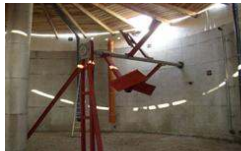
Digester inside view
