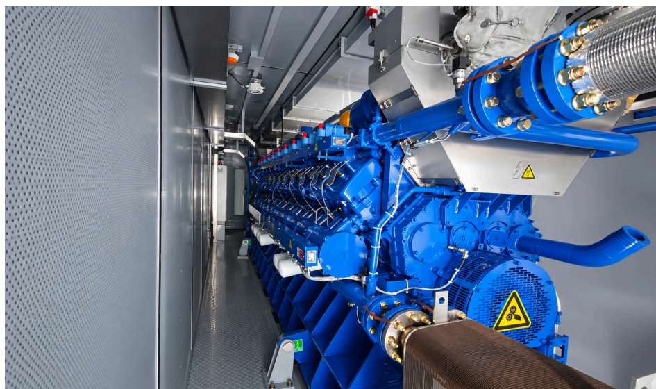
Internal view: engine, alternator and service access
