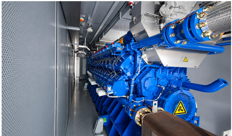
Engine compartment and service access
