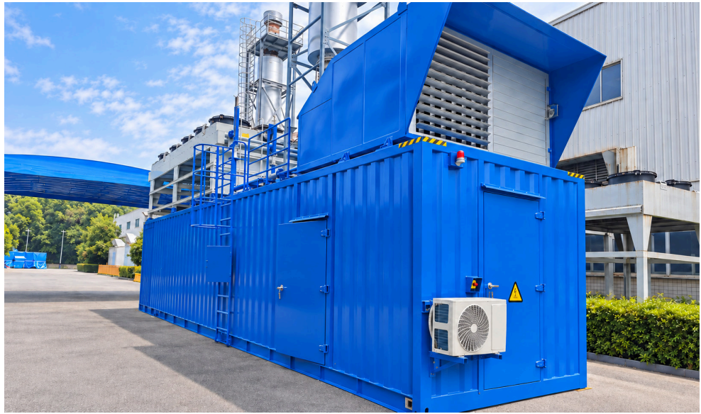
Container, cooling and ventilation equipment
